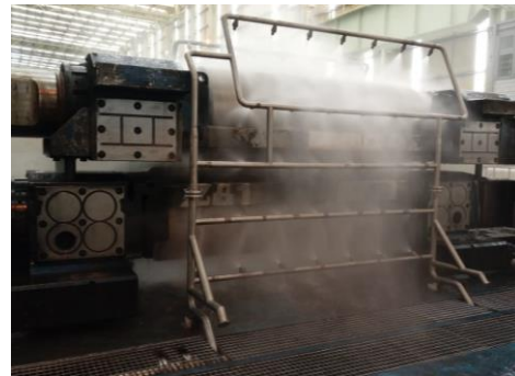
Figure 3: New cooling system device
