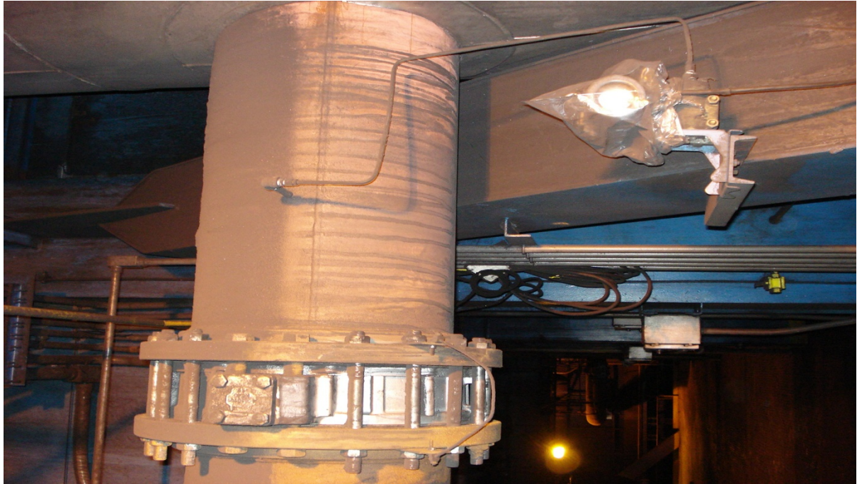
Figure 6 - Inlet suction pressure transmitter
