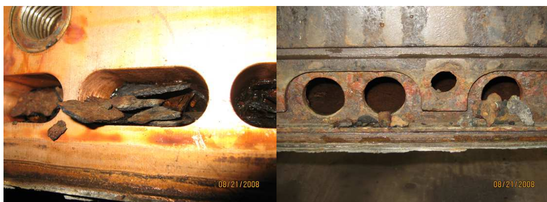
Figures 6 and 7: Scale blockage in connecting holes of a high speed copper and Scale in water jacket water feed ports
