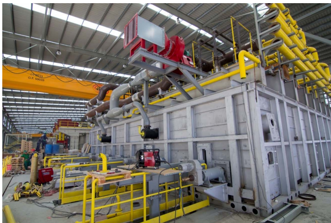
Figure 3: Billet Reheat Furnace
