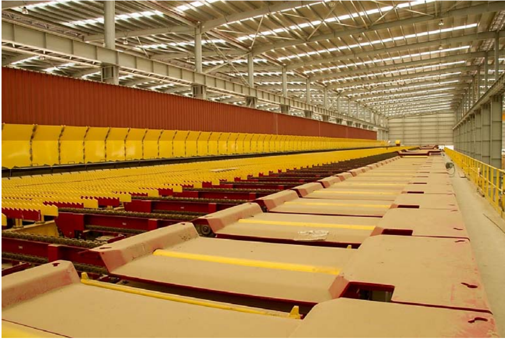
Figure 5: Cooling Bed and its Exit Roller Table
