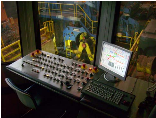
Figure 2 - View from the pulpit of downcoiler in operation
