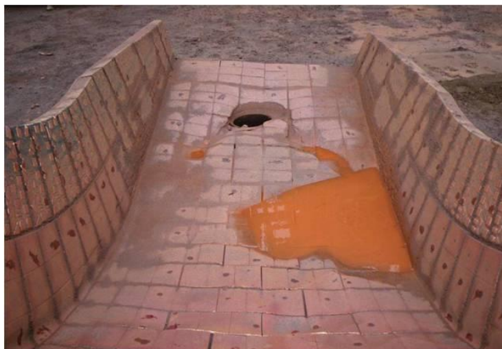
Figure 3. Impact plate showing wear.
