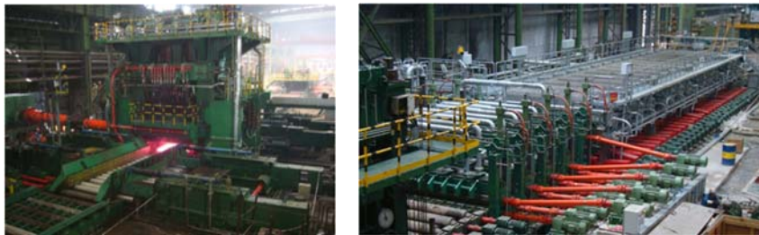
Fig. 3: Modernized 4-high finishing mill stand in operation (l), new plate cooling system (r)
