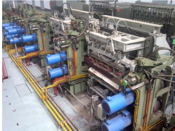
Figure 10. Induction heaters by ABP Induction Sys
