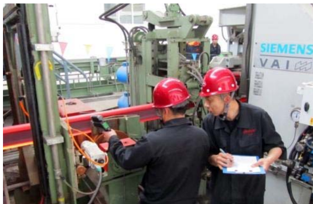
Figure 23 Temperature measurements during commissioning
