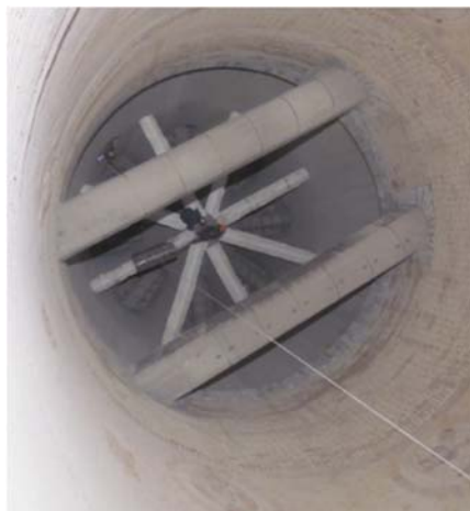
Figure 4: The AGD in place at COREX ® Baosteel Module 02
