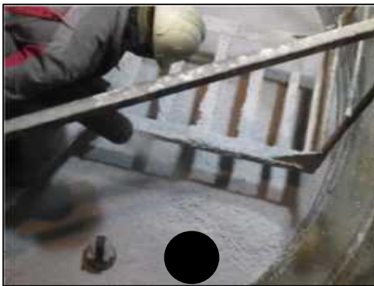
Fig.5. A: casting on site the bottom B: Using precast segments for the safety lining
