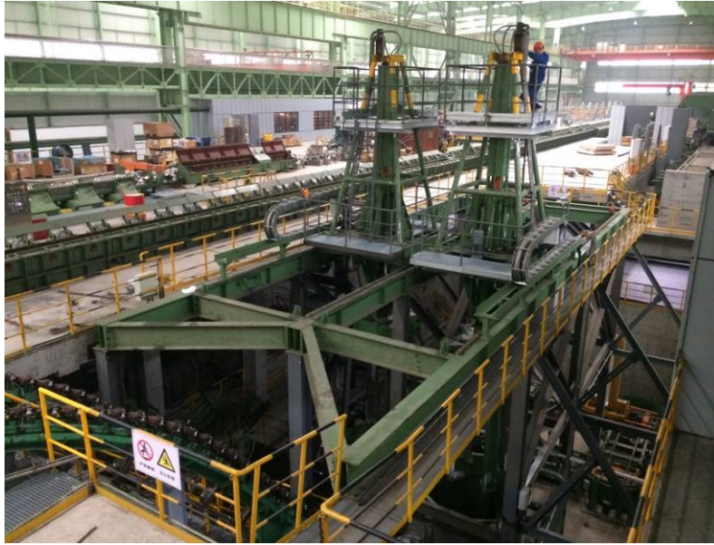
Figure 11 - Pouring Reel Outlet with Water Quenching Tanks
