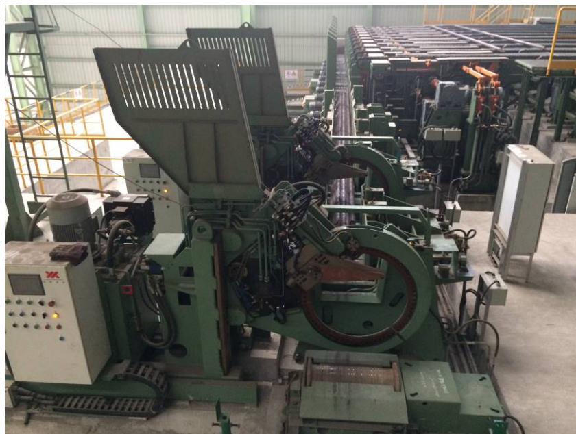
Figure 5 - Bundling Station & Tying Machines
