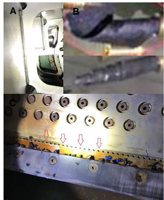
Figure 13. Photos showing the inside of the HTRC (A), the blocked HTRC nozzles (B), caused by pieces of plastic and oxide particles (C).
