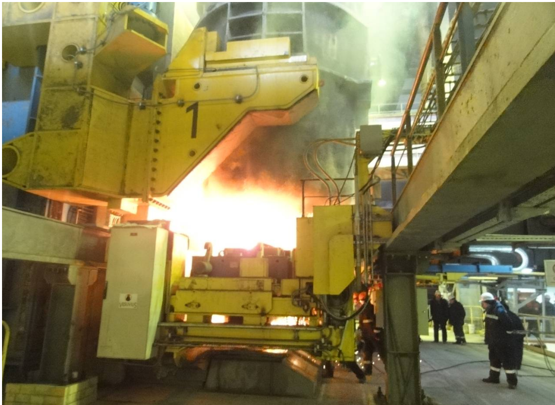
Figure 5 - Ladle turret plant view.
