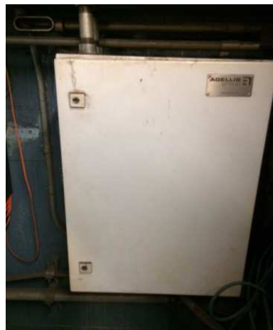
Fig. 11 Control unit on the casting floor
