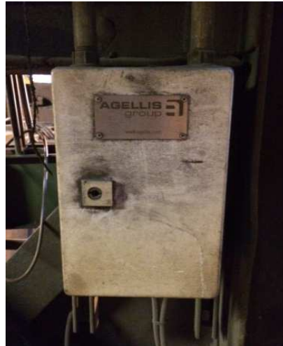
Fig. 10 Pre-amplifier unit on the casting floor
