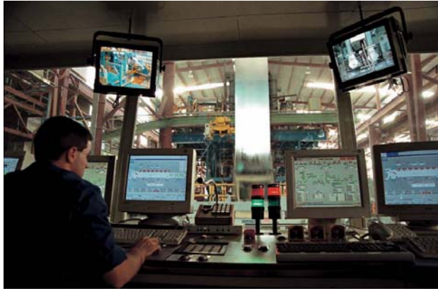
Figure 9. Process control pulpit.
