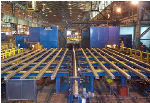
Figure 6. Billet surface conditioning plant
