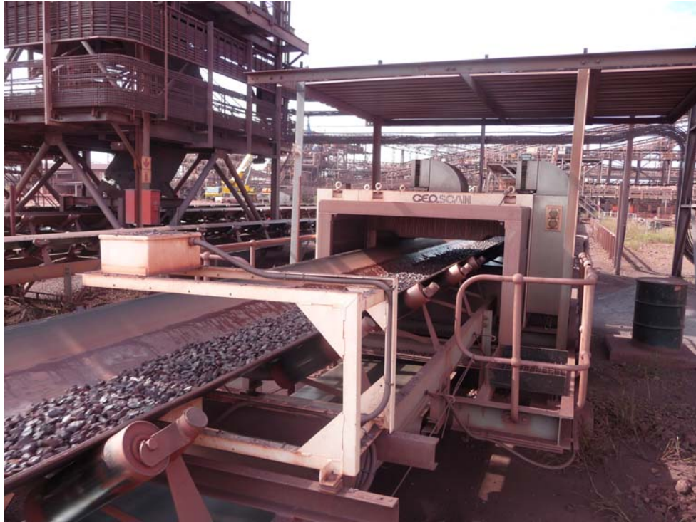
Figure 5. Elemental and moisture analyser installation in iron ore beneficiation plant.
