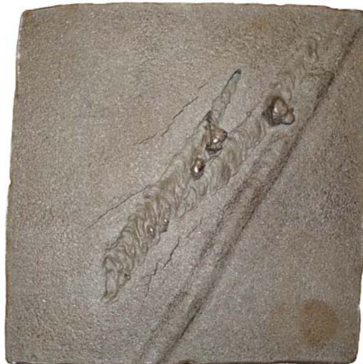
Figure 1: Steel Shell damaged by SCC - Interior of the repaired area
