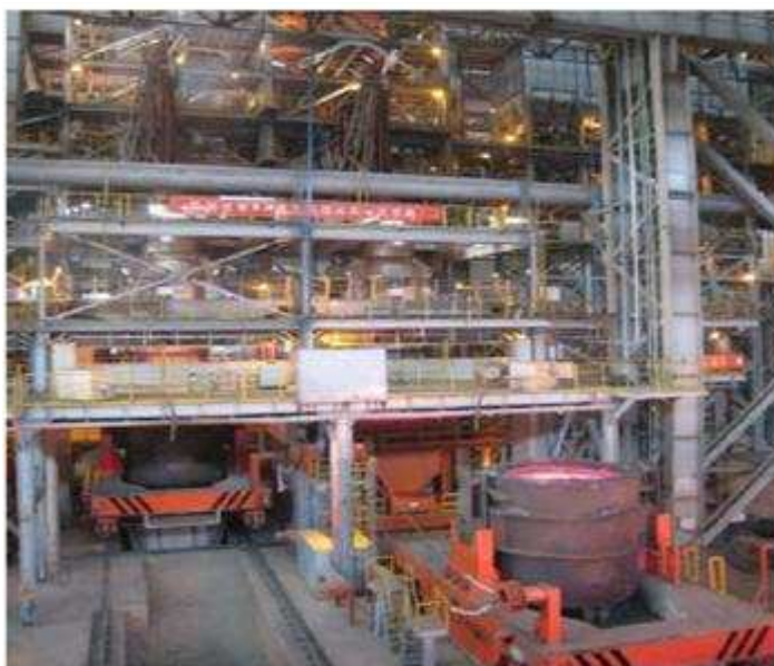
Figure 8. Twin Stand RH Plant at Nanjing ISCO.
