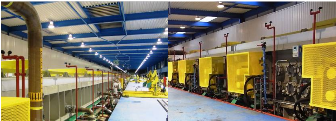
Figure 6. Example of modernized equipment (pickling and rinsing tanks).
