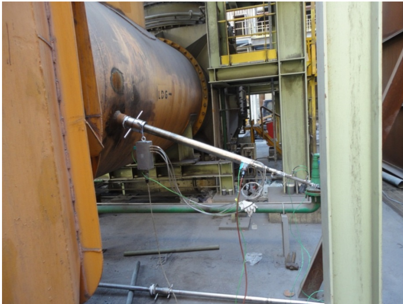
Figure 2. Typical setup for a measurement location at outlet of ID Fan.
