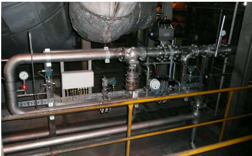
Figure 4. Compact oxygen flow train installed on the walking beam furnace at SSAB, Borlänge in Sweden.
