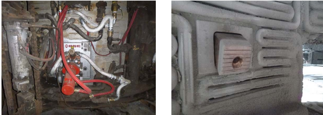
Figure 2: Exterior view of installed tiltable VLB (left) and interior view (right) in a side-wall panel
