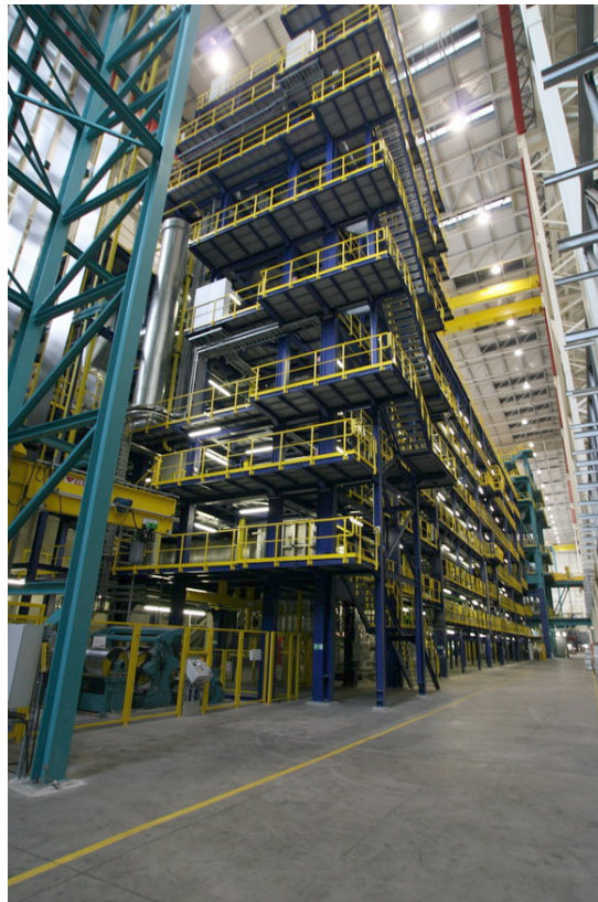
Figure 6: Furnace CGL no. 4.
