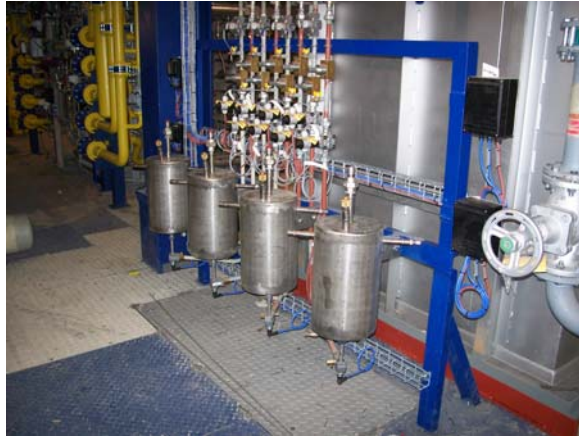
Figure 10: DFF Waste Gas Analyzer Station.
