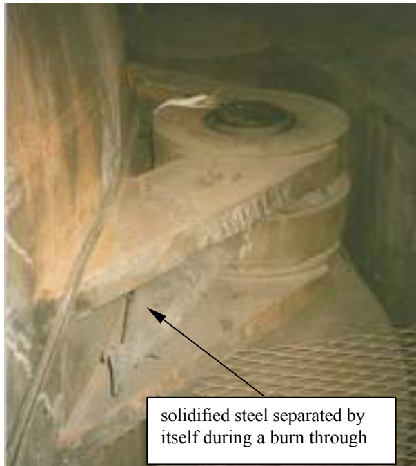
Figure 13: Solidified liquid steel on horizontal link arrangement after a burn-through
