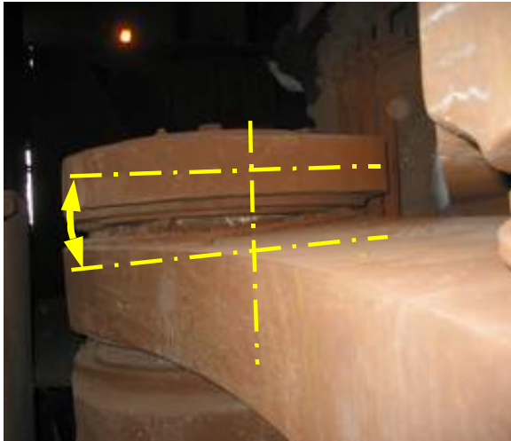
Figure 9: Horizontal link with swivelled link showing the function of the spherical plain bearing
