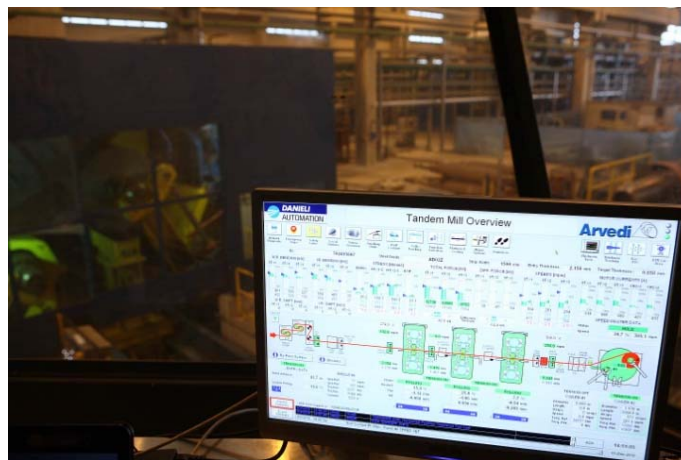
Figure 7: HMI Tandem Cold Mill
