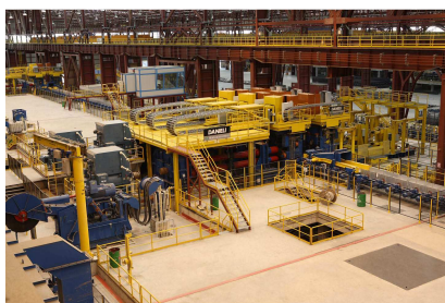
Figure 6 - Commissioning of medium section mill at Siderurgica Balboa (Spain).
