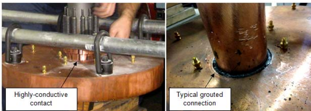
Figure 3. Finger cooler installation (left) and cigar cooler installation (right)
