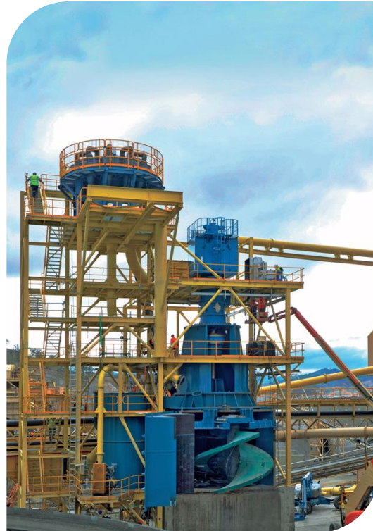
Figure 5: Cadia's VTM-3000 (Tertiary Grinding Stage).
