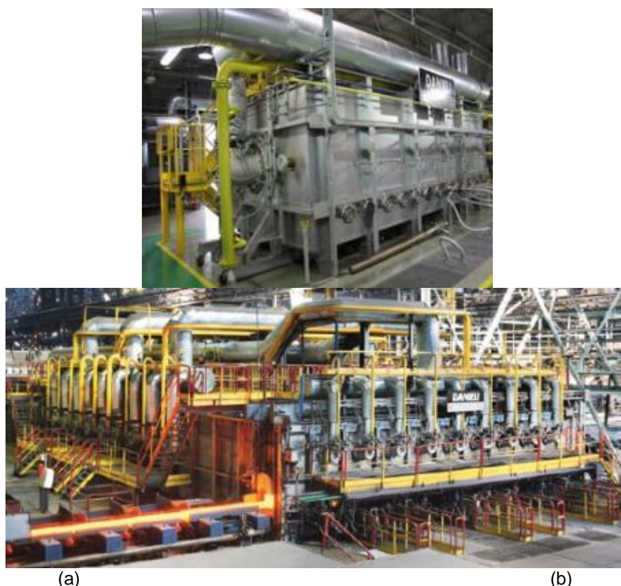
Figure 3. (a) pilot plant at Danieli Centro Combustion Research Center (Savona, Italy), (b) plant walking-hearth RHF
