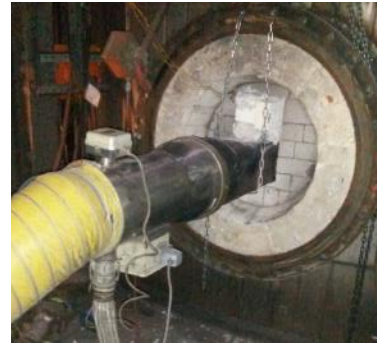
Fig. 11 – NG burner for re-heating
