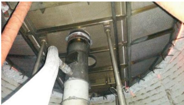
Fig. 9 – Burner in position
