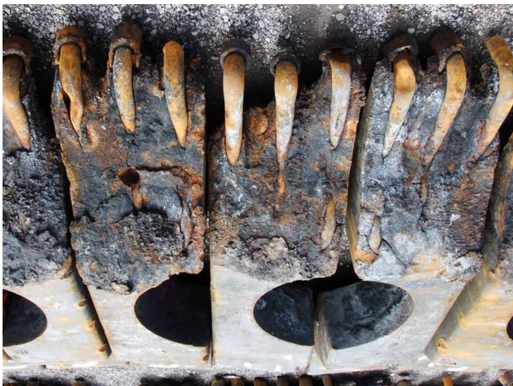
Fig. 2 Worn out tuyère staves after dismanteling
