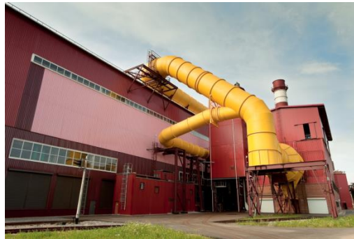
Figure 1: Secondary Gas Cleaning System
