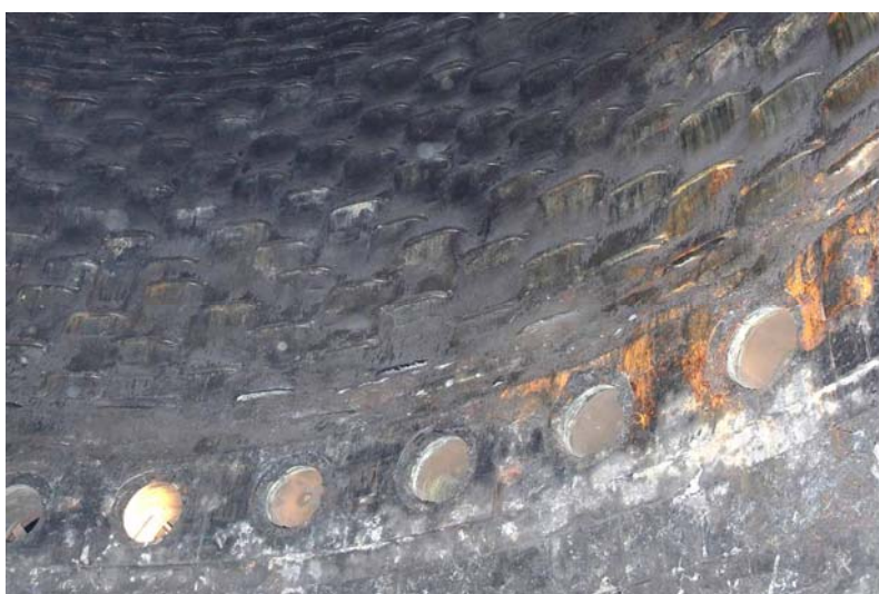
Figure 3. IJmuiden No. 7 bosh condition after 15 years in operation.
