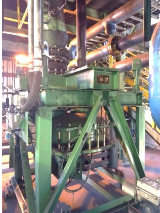
Figure 2. Solid pulverized fuel feeding system.
