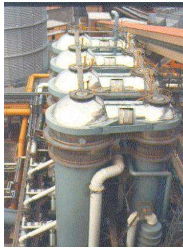
External Combustion Chamber Stoves
