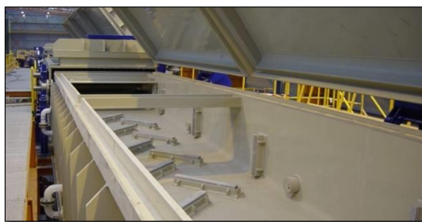
Figure 3. Polypropylene pickling tanks
