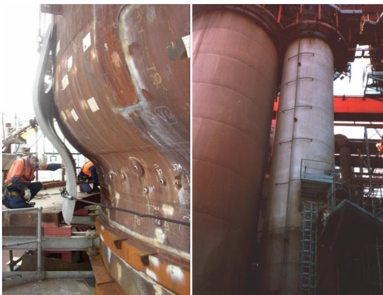
Fig. 5: (left side) Double shell during erection on a stove dome, (right side) Double shell after completion on a stove combustion chamber
