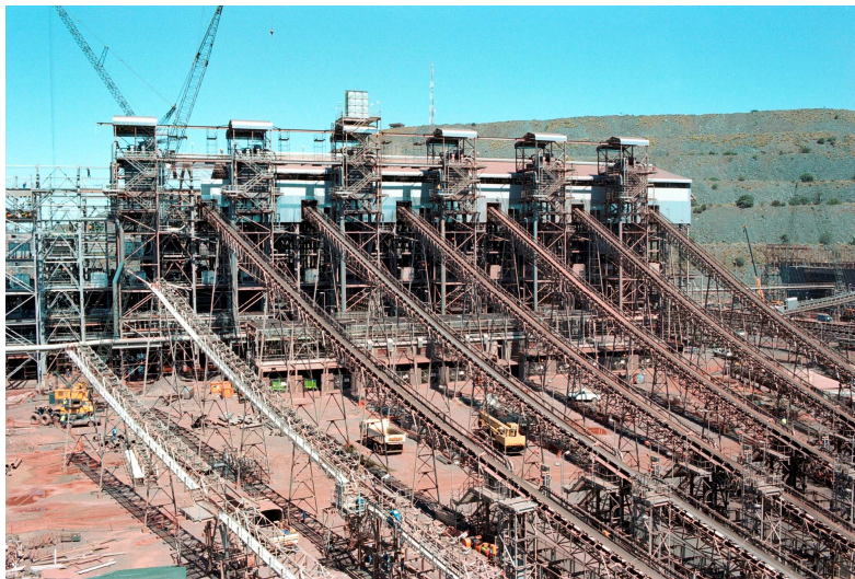
Figure 4: Iron ore jig plant, Sishen, South Africa.
