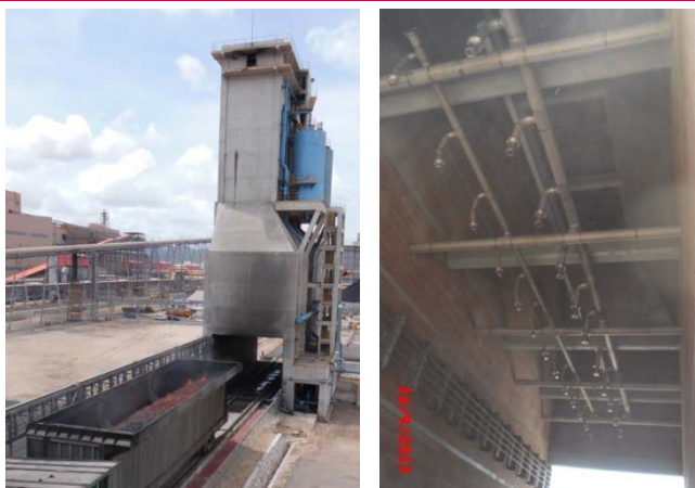
Figure 5 Quenching tower and spraying nozzles
