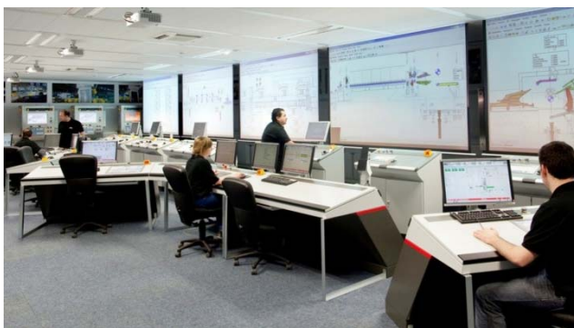
Figure 16: Plug & Work Test: original automation equipment including operation desks and stations in the test field
