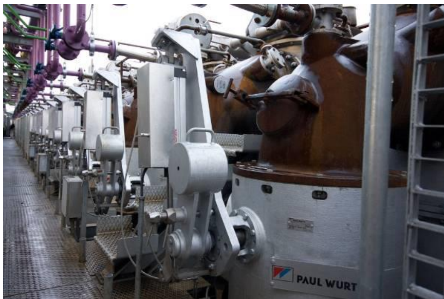
Figure 9. SOPRECO® valves installed in ZKS coke oven batteries.
