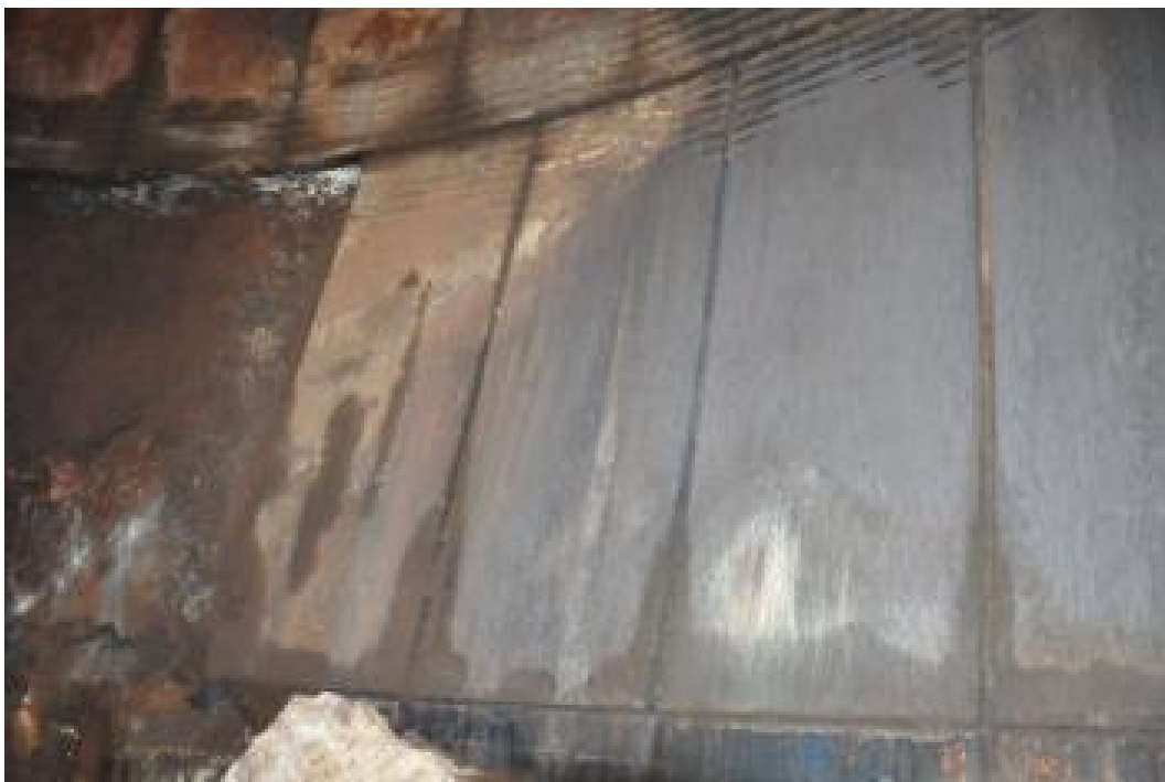
Figure 6. Stave condition after the blow-down.
